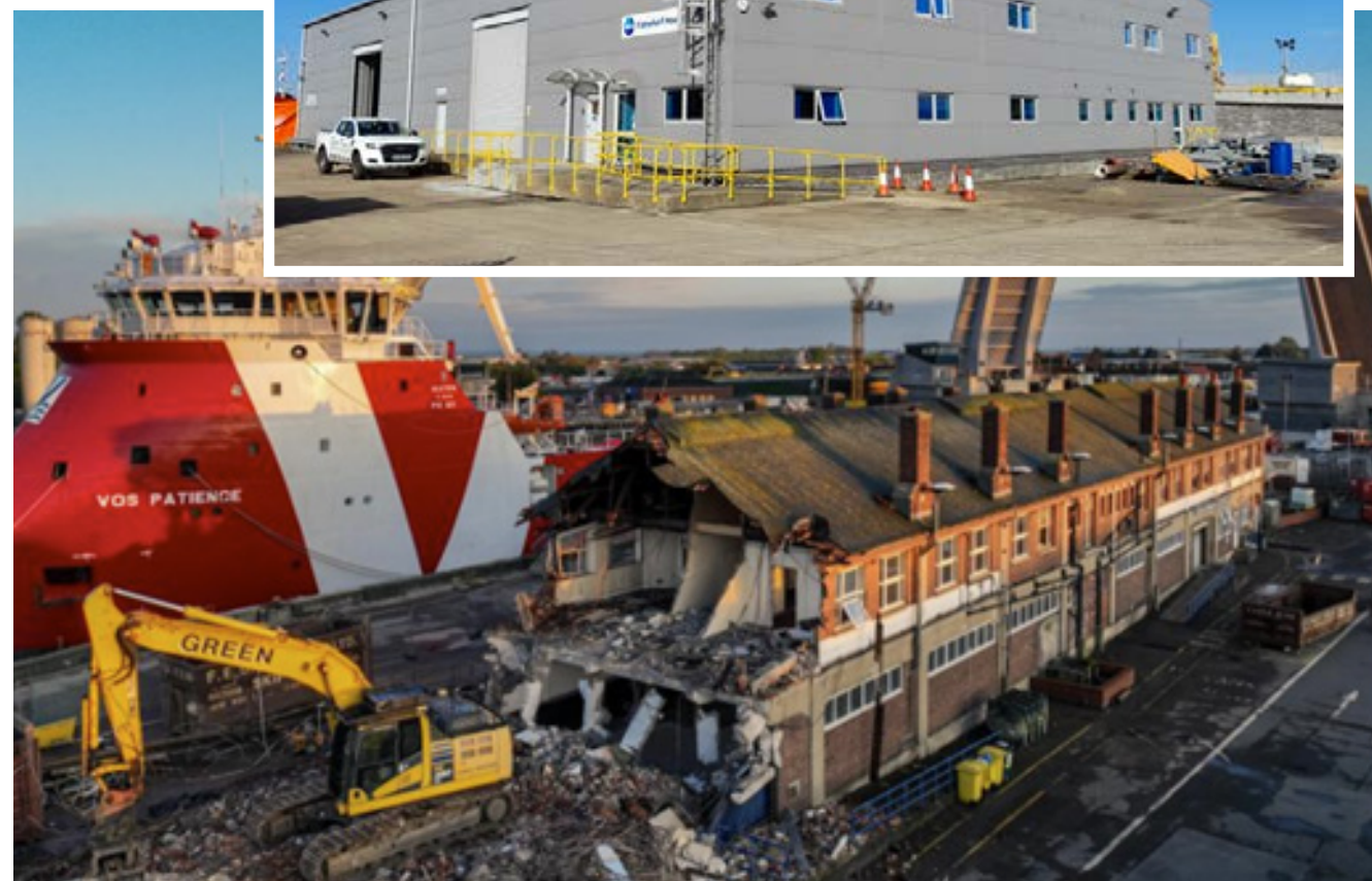
Redevelopment of ASCO base in Great Yarmouth, UK, to include new offices, enhance laydown space and provide ship-to-shore waste capability.
